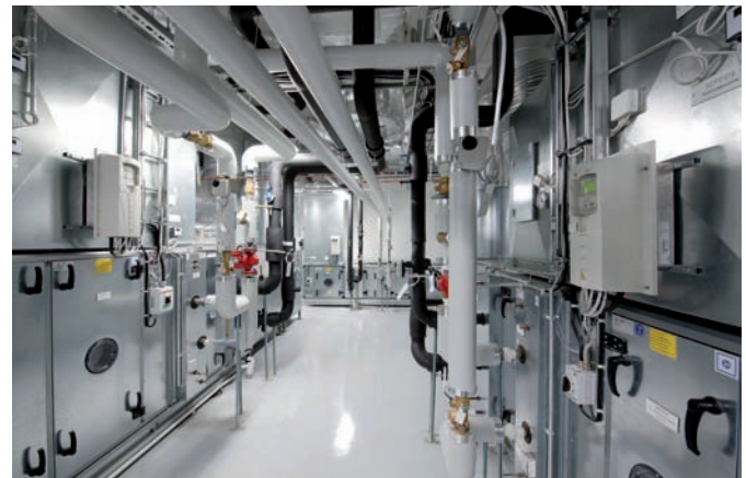
BACnet-based HVAC system controls air quality at ABB's Vuosaari factory, while also assisting with functional testing of ABB's Azipod® marine propulsion units.
