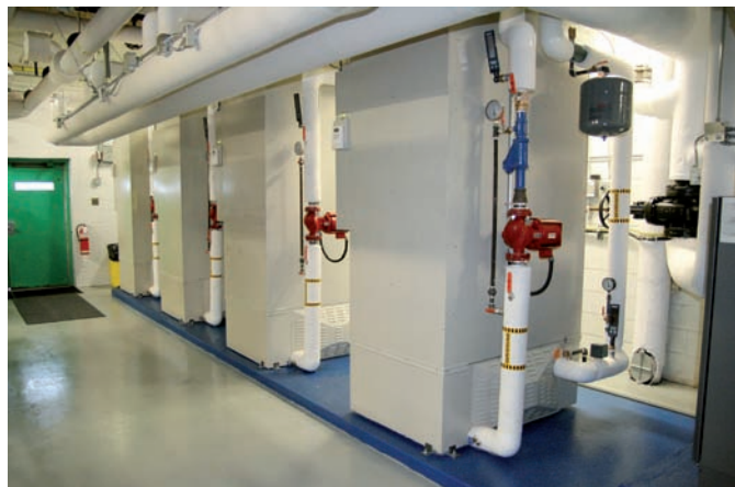
Mechanical room at St-Roch-de-L'Achigan School.
