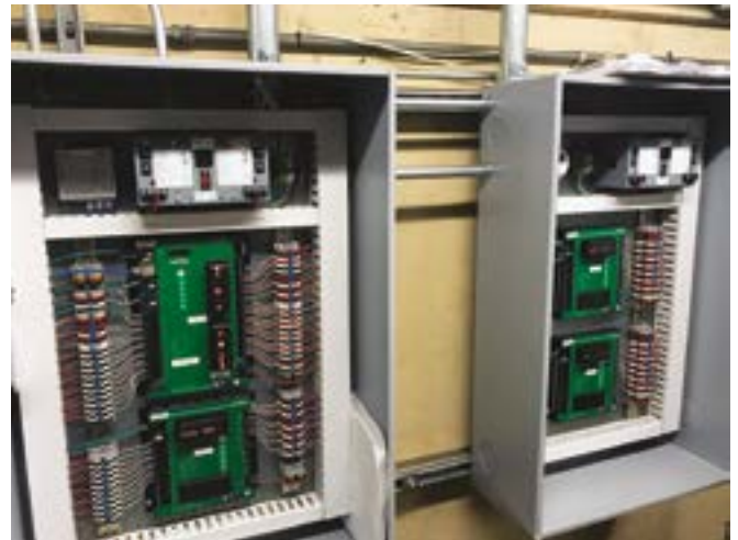
BACnet control was provided by the Conquest line © Comfort International by KMC Controls, Inc.
