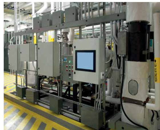
Mechanical room at MaRS. © Modern Niagara Group Inc.
