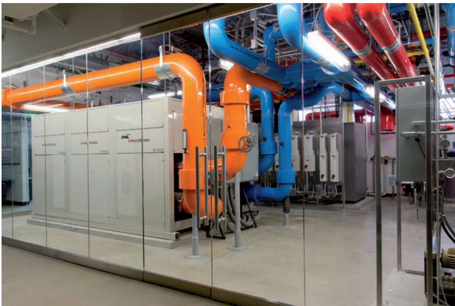
The HVAC System is critical for manufacturing and reliability
