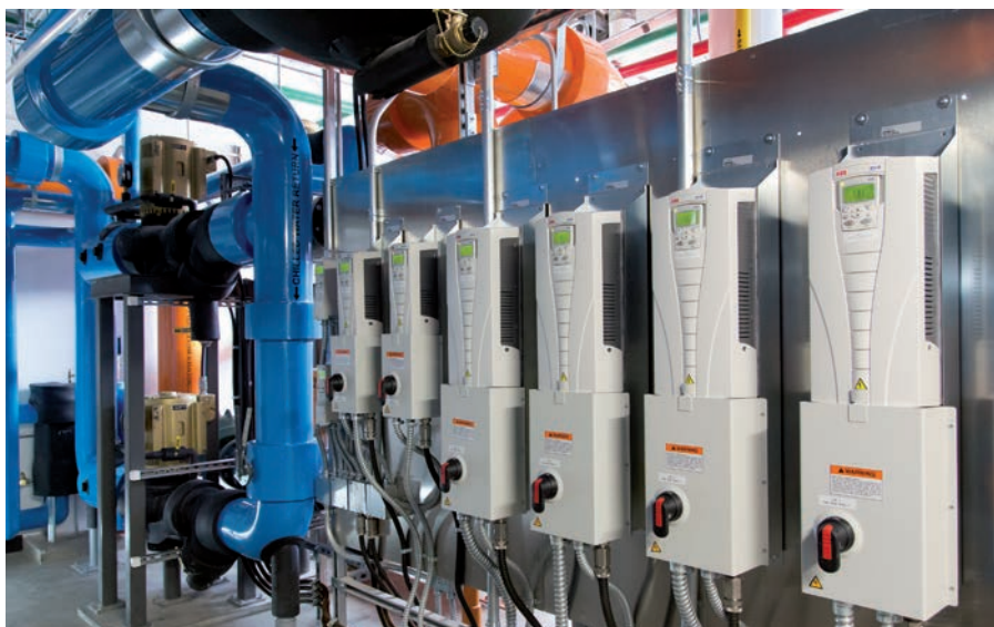
Nearly every device in the highly intelligent and flexible building communicates via BACnet
